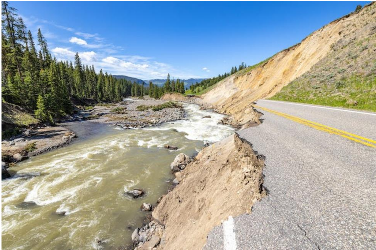
Fast-moving floodwater obliterated sections of major roads through Yellowstone National Park in June 2022. Jacob W. Frank/National Park Service
