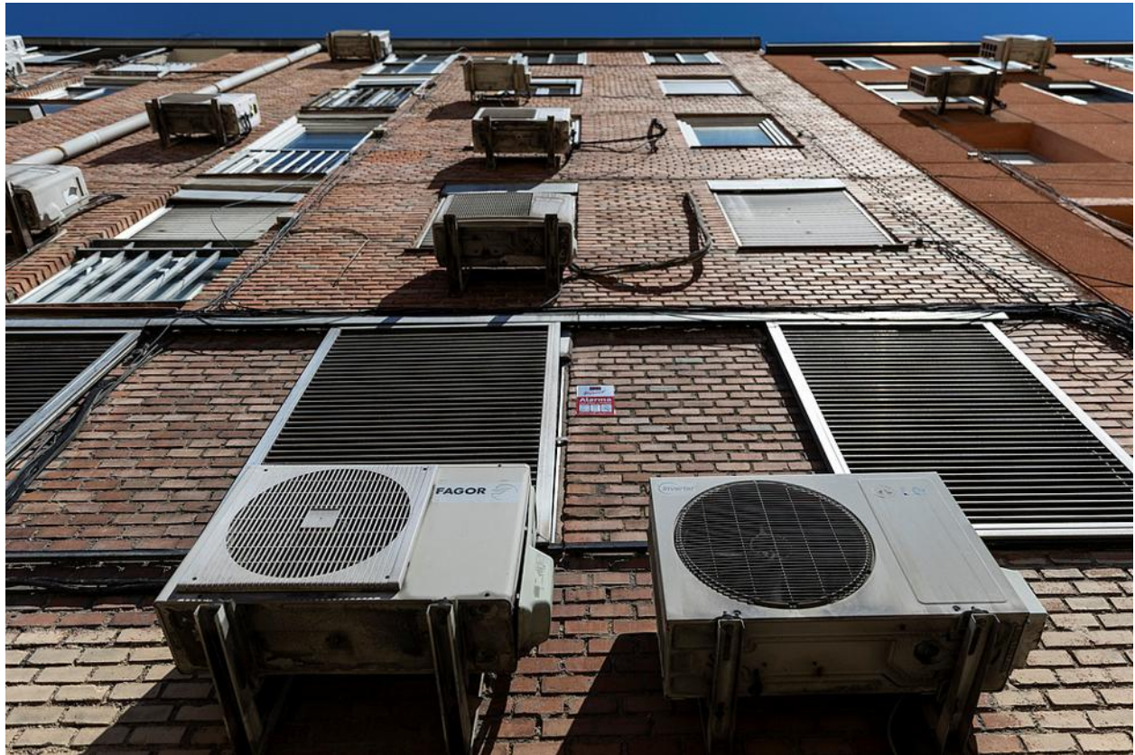
Air-conditioning units are installed on the exterior of an apartment building in Madrid, Spain, May 23, 2026. /CFP
